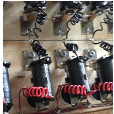
Close up of magnets, cabling, and bus bar inside Gamba wind chest
